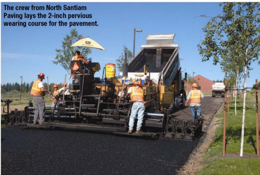
A geotextile fabric was laid on top of the porous asphalt pavement to keep fines out of the road structure during construction of the community.
