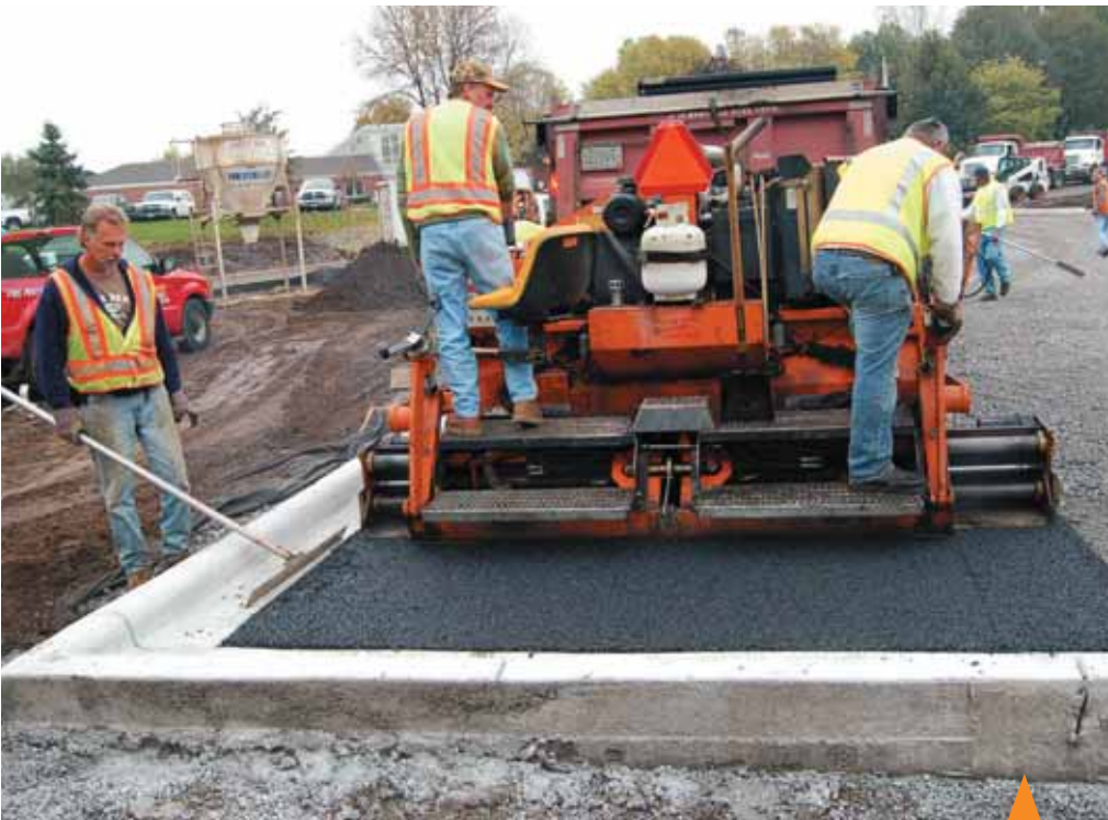
The crew of Pine Bend Paving begins to lay the mat for a porous asphalt parking lot for the Ramsey-Washington Metro Water District in suburban Minneapolis-St. Paul. (Photos courtesy of Barr Engineering and Pavement Management Services.)
