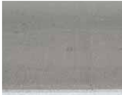
Transverse tined PCC pavements like this one can make traffic noise very loud for local residents.
